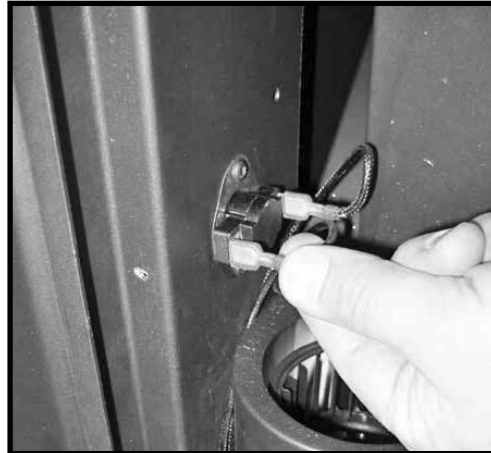
Figure 14: Disconnecting thermal switch.
