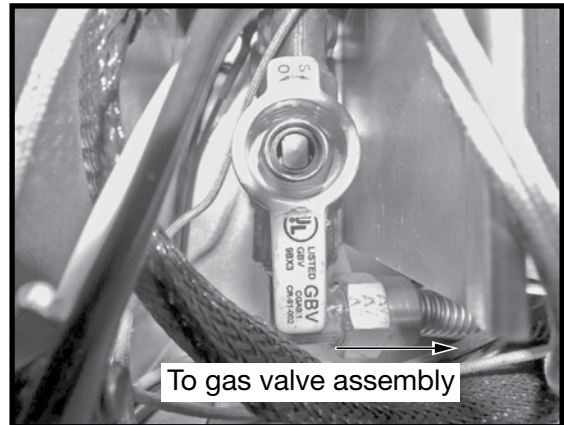
Figure 35: Gas shut off valve.
