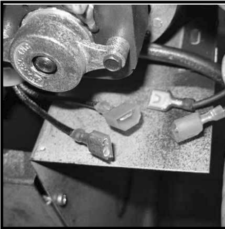
Figure 13: Disconnecting fan wires.
