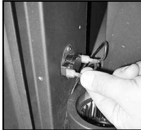
Figure 14: Disconnecting thermal switch.
